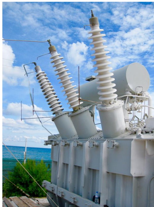
Figure [12]. Coated bushings at coastal test station in Greece.
