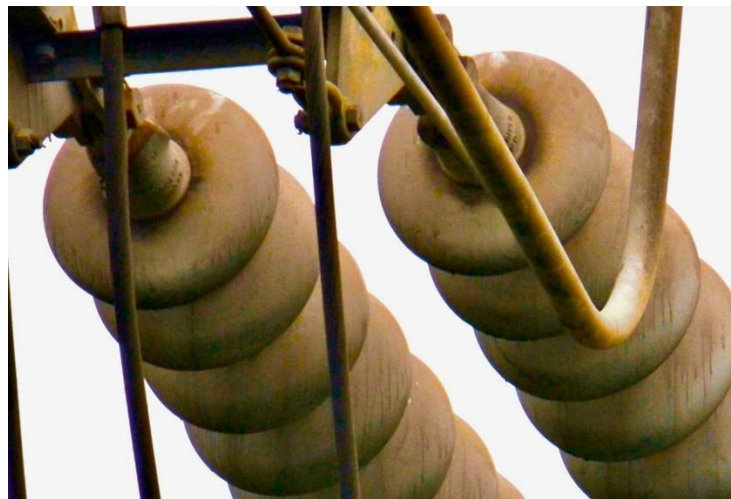
Figure [19]. Degradation of coating at line end of coated string.
