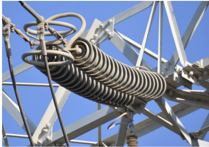
Figure [4]. RTV-coated glass string on transmission line in Italy.
