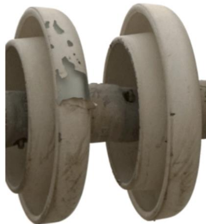
Figure [2]. Example of peeling of RTV coating.
