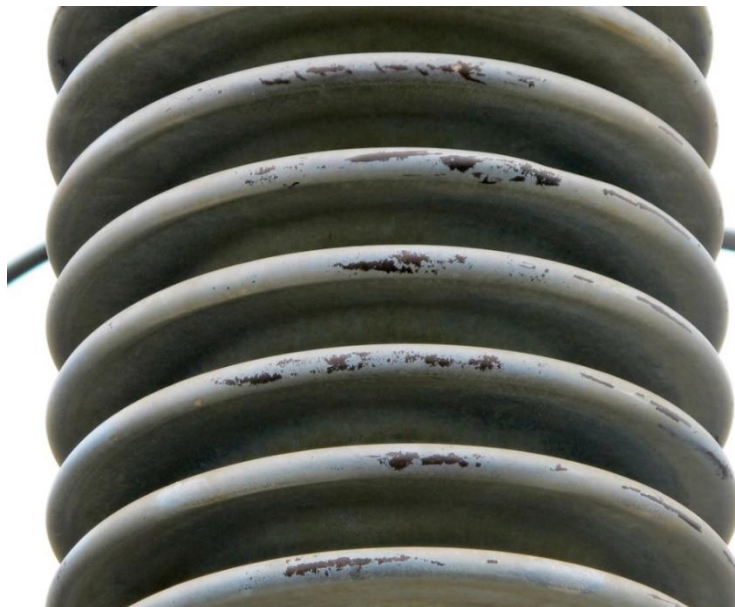
Figure [18]. Evidence of end-of-life of coating at polluted substation in China.
