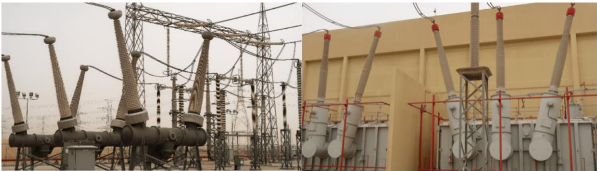
Figure [6]. Station insulators coated with RTV at Al Fadhili back-to-back converter station.
